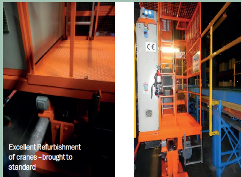
Figure 10.33: Improvements through restoration – examples of a crane after refurbishment works (asset care step 5b)
